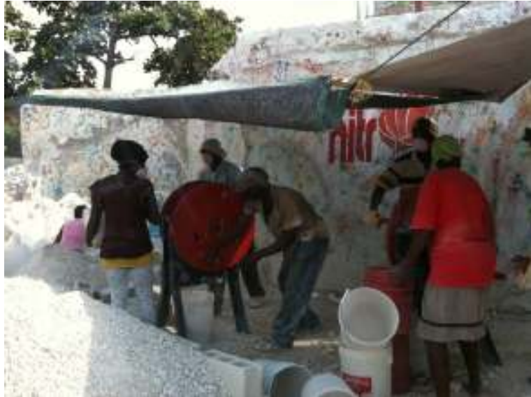
R2R entrepreneur and work crew crushing rubble at a CRS Community Resettlement and Recovery Program site in Christ Roi. Photo: Kevin Osborne.
